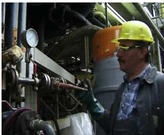
Figure 11: SF 6 re-use in gas manufacturer installation
